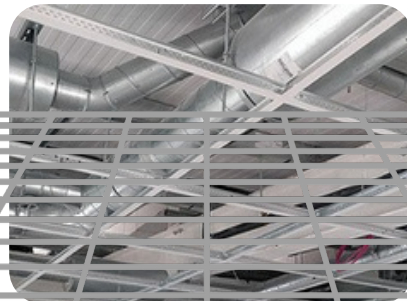
Suspended ceiling grid
