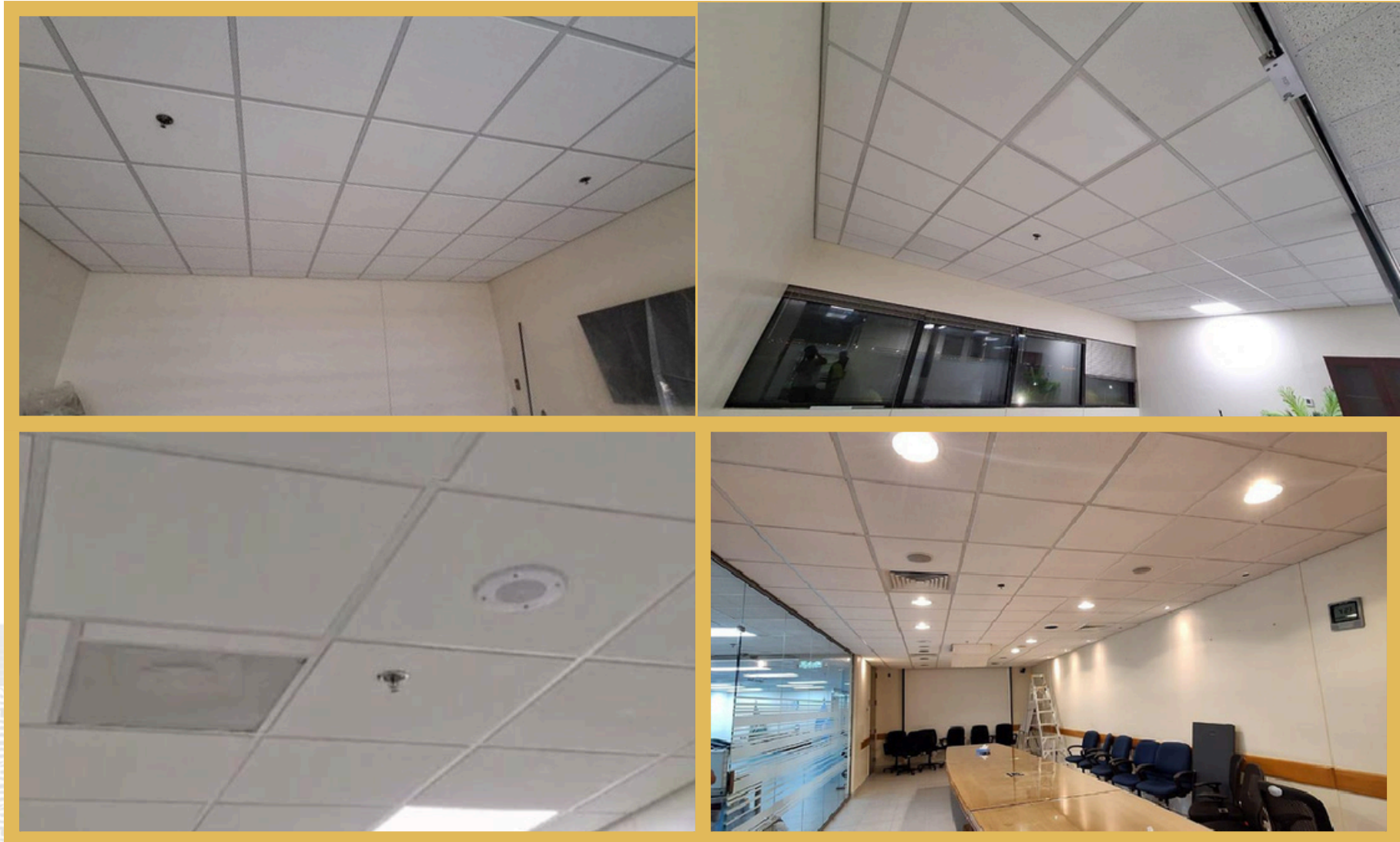
SUSPENDED CEILING GRID (CATRION)
